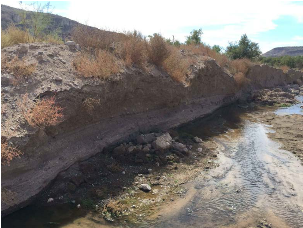
Photo 18. Meadow Valley Wash – Bank Erosion Downstream Southwest U.S. Highway 93 Bridge
